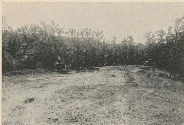
THE 14TH GREEN UNDER CONSTRUCTION Requiring a great deal of cutting and filling
